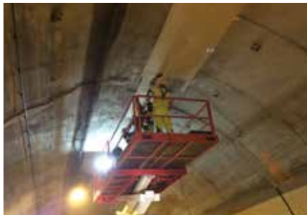
The fire-protection boards were installed onto the tunnel ceiling from lifting platforms. Inspection: Täby Brandskyddsteknik AB
