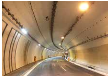
Finally, the walls received a structural lining on top of which the fire-protection cladding was mounted. Inspection: Täby Brandskyddsteknik AB
